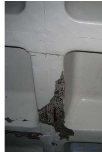
Figure 17: Section of the waffle slab that was contained spalling concrete with rebar exposure.
